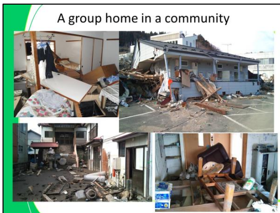
Figure 12 Corporation building damage: group home
